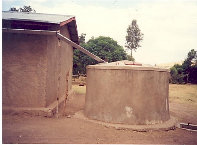
Figure1: Roof top water harvesting and storage system
