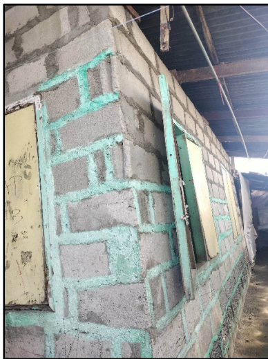
Fig. 7 Bad Construction. No Supported Columns and Beams
