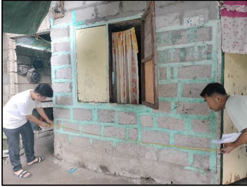
Fig. 3 The length of every wall in the house was not more than three times the width. Image from Model Community, Porac, Pampanga
