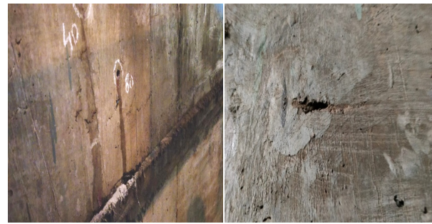
Fig. 5: Honeycombed Concrete observed
