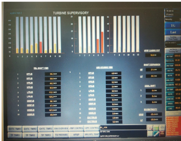
Figure 10: TG deck Vibration data before restoration
