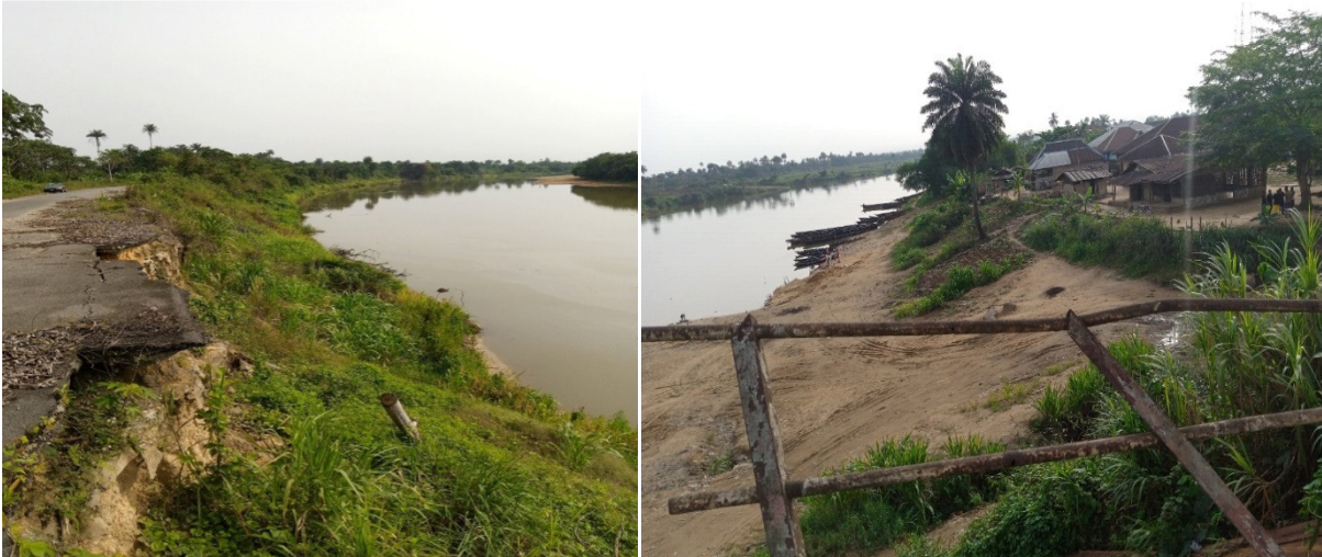
Plates 1. (A & B): Deplorable road embankment due to shoreline change along Joinkrama road and Riparian dwellers proximal to the shoreline under study Area.
